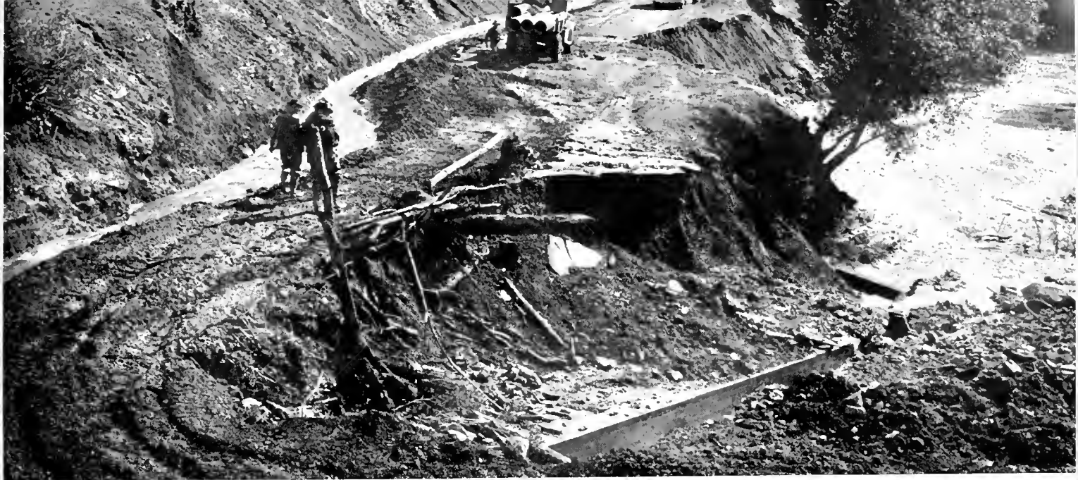
Washout on U. S. 299 West of Redding caused by February storms. Large sections of pavement were destroyed by undermining waters
